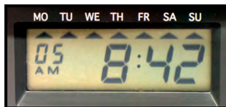
Figure 7-8: Failed Time Synchronization Display
